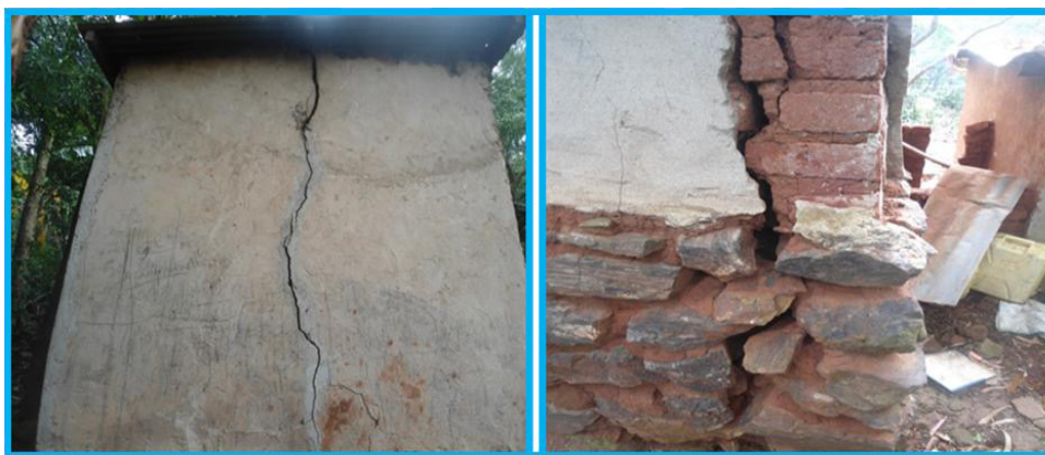
Picture 6.18: Some cracks on the walls on the house of one of the Katoma street resident alleged to have been caused by blasts and vibrations from GGM mining areas.
