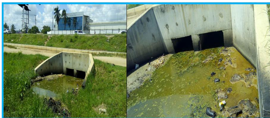
Picture 6.22: Waste water allegedly from the Chemicotex Industry. The waste water was passing under the road to surrounding communities as seen in the picture.
